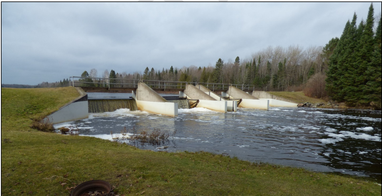
The Presque Isle Wildlife Dam south of the community of Marenisco, in Marenisco Township, was repaired after flooding in 2002 and 2013. Wakefield Township is at minor risk of flood impacts from a future failure.
